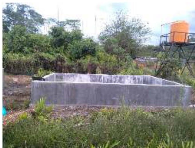
Figure 2. Water storage tank
