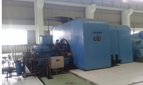
Gambar 6. Condensat Extraction Steam Turbine
